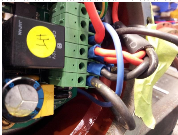
Retrofit kit wiring connected to the PCB
