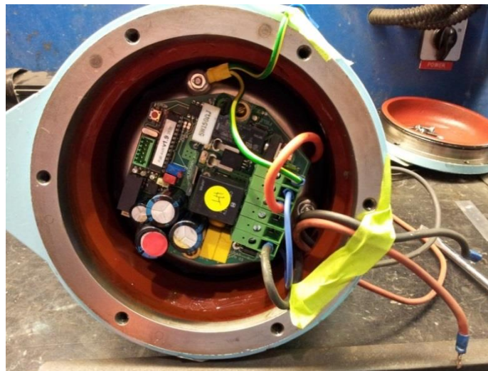
Alternator with rear cover removed, load wiring disconnected and tethered out of the way
