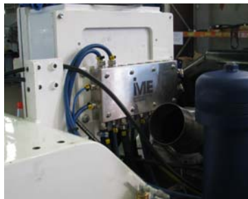
I.S. junction box, often mounted directly behind the FLP enclosure
